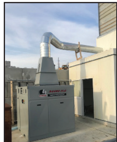
Aggre-Flo heater installed at a precast plant
